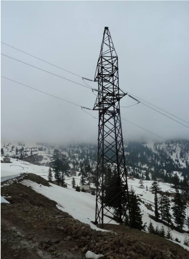
Figure 2.12: Existing 110 kV transmission line
