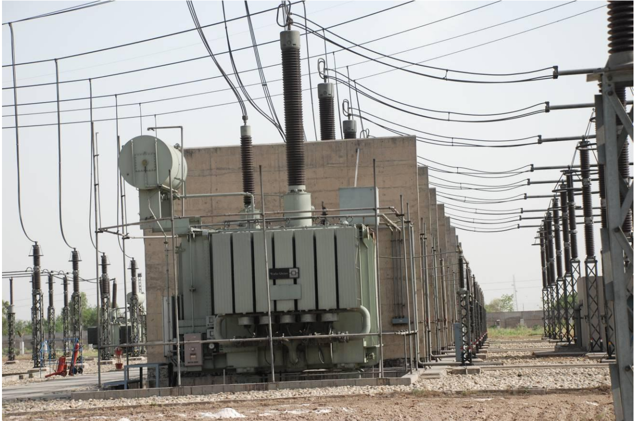
Figure 2.11: Example of Transformer and Switchyard location
