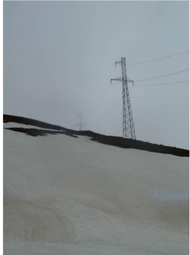
Figure 2.13: Existing 110 kV transmission line
