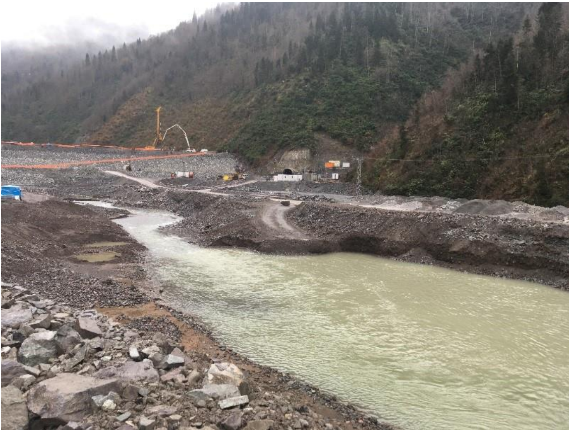
Figure 10: Over widened reach 300 metres downstream of Skhalta dam which will require narrowing prior to commissioning
