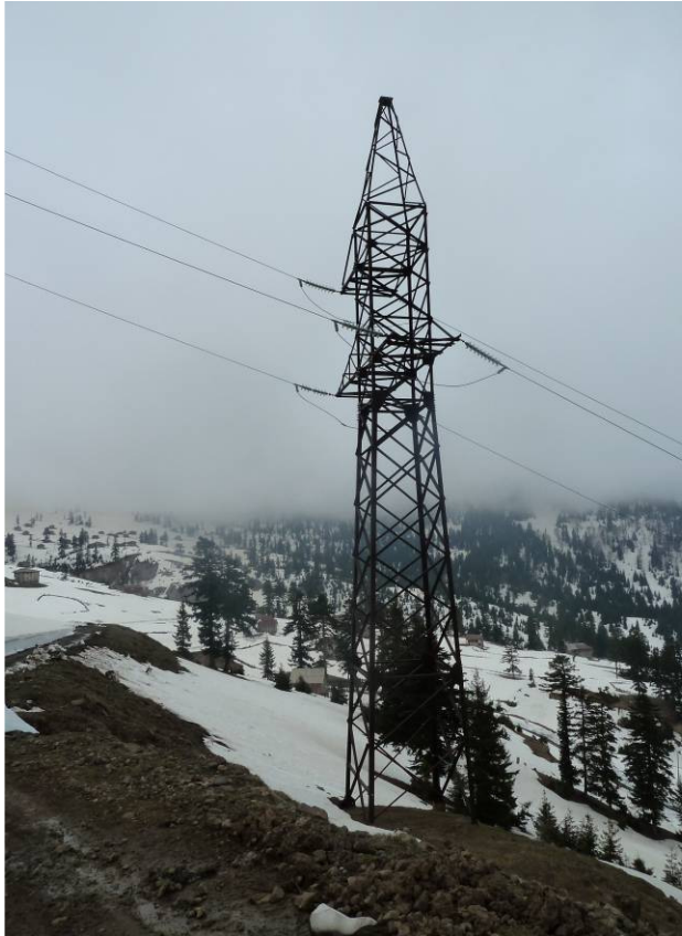
Figure 2.14: Existing 110 kV transmission line
