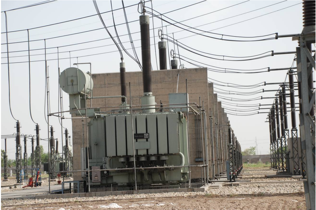
Figure 2.13: Example of Transformer and Switchyard location
