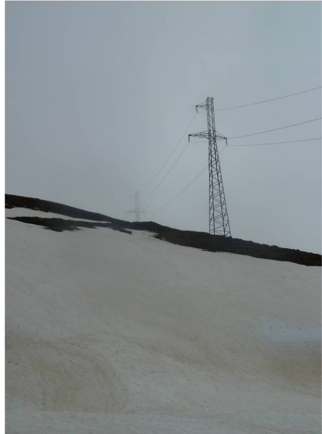
Figure 2.15: Existing 110 kV transmission line
